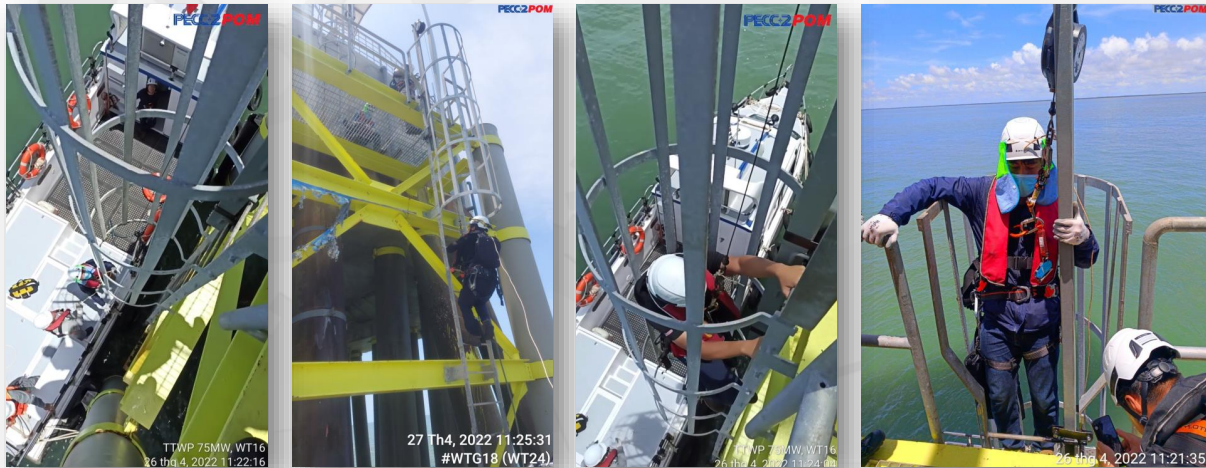
Access wind turbines for maintenance
